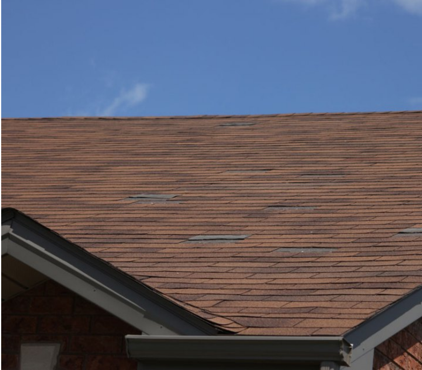
Missing shingles can be seen on this rooftop. (RICK DAWES / The Windsor Star)
